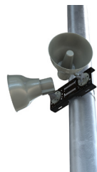
Dual Paging Horn installation
